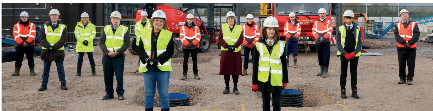
Staff and students of Castell Alun High School at the monumental steel beam signing ceremony.
